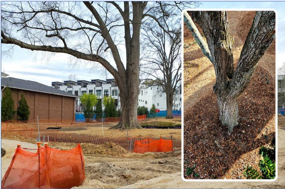
Existing (legacy) trees were protected during construction activities and invigorated with air spading and the application of a compost/sand blend (inset). Photos by Ron Alexander
