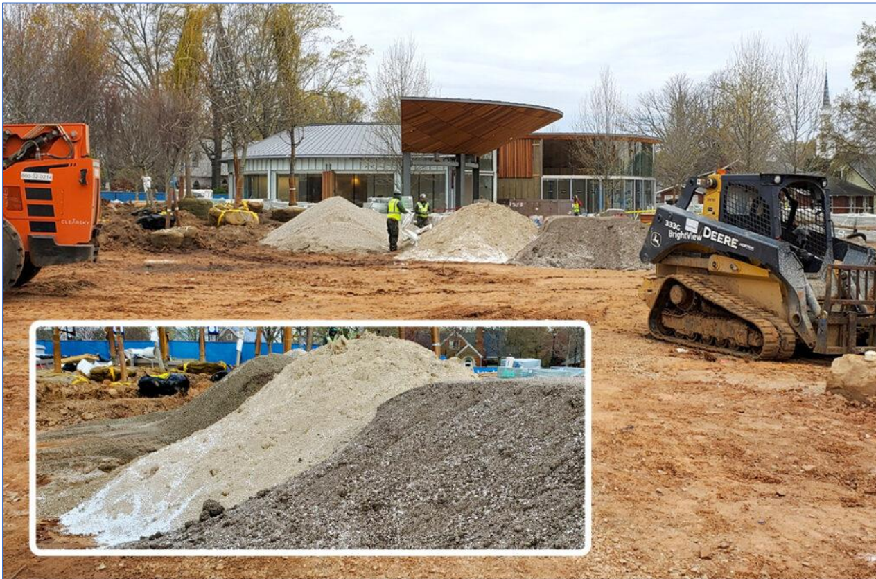
Dense, clay-based soil native to the Piedmont region of North Carolina was improved with engineered soils containing compost for planting areas and bioretention features (inset). Photo by Ron Alexander and inset courtesy Wade Moore Equipment
