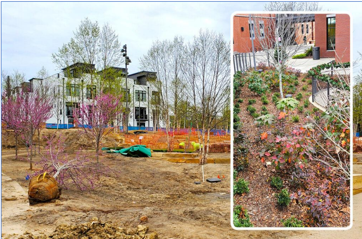
New planting area for trees and shrubs (inset), established in engineered soils containing compost. Photos by Ron Alexander
