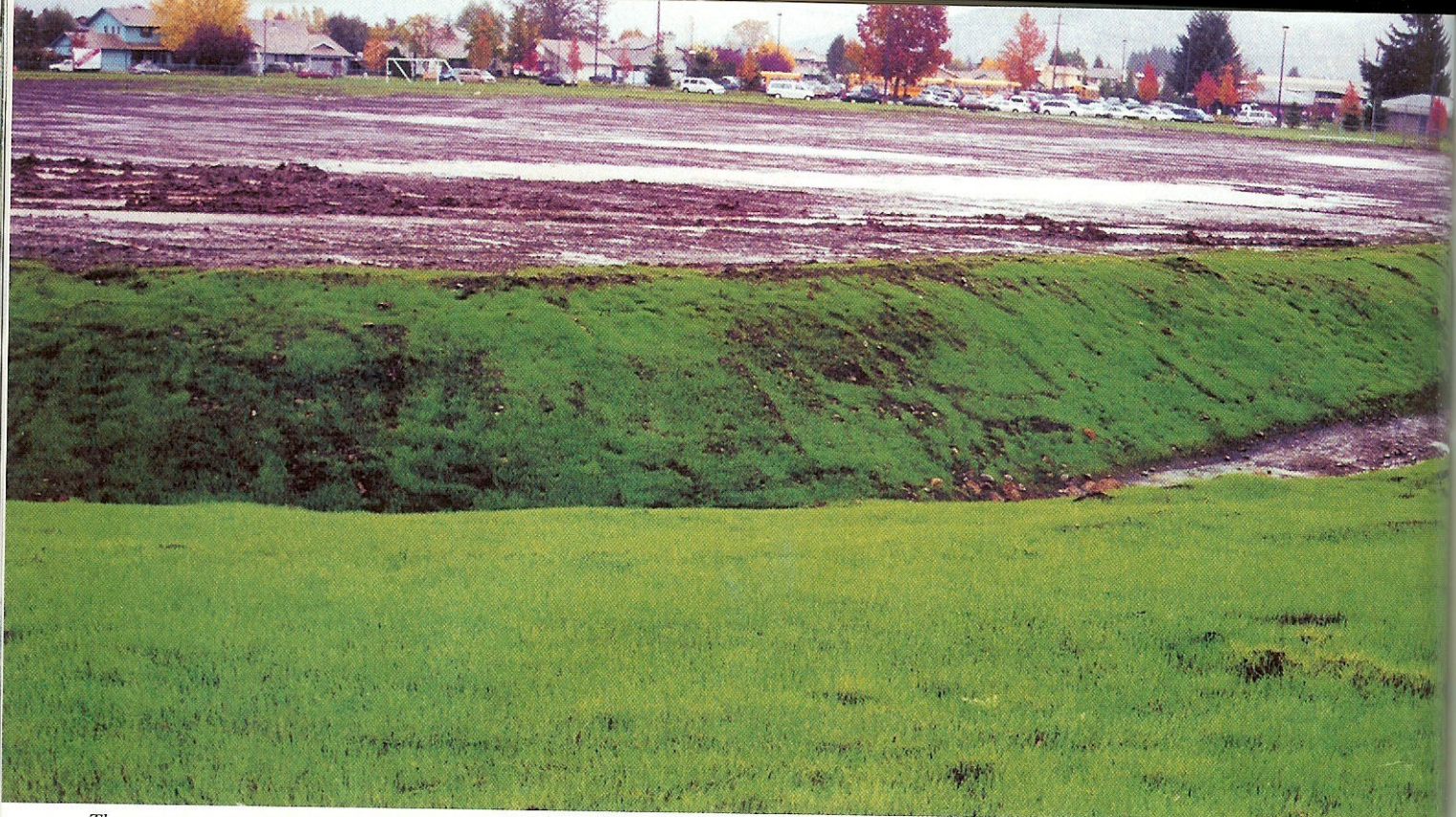
The compost was pneumatically applied along with seed on the waterway slopes. The benefits of using compost-based techniques such as hydroseeding, straw mulching, erosion blankets and geotextiles, hay bales and sediment dams include: immediate and effective control, they bind and degrade specific chemical contaminants, and help in the efficient establishment of vegetative cover.
